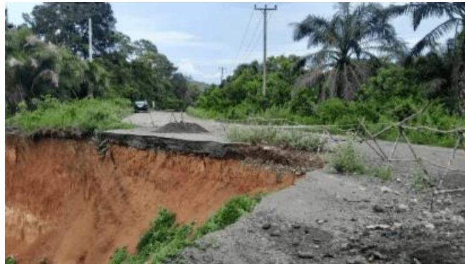
Figure 1. The road conditions in Urai village are broken due to abrasion.
