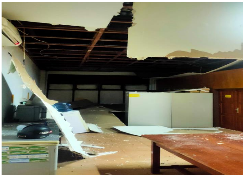
Figure 1. Moderate damage to the agricultural lab building at Halu Oleo University
